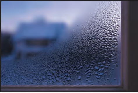
Condensation on the inside of a window-pane.
